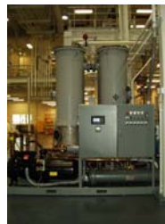
CE-500 Evaporator treating low level radioactive wastewater
